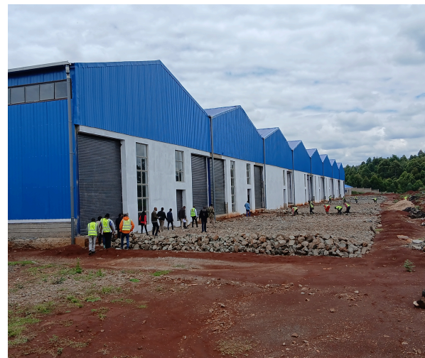
Kiambu County Aggregation and Industrial Park at Githunguri stands at 75% completion. The CAIP will focus on coffee, dairy and pineapple for value addition.
